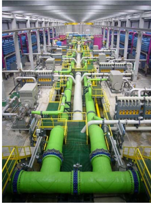
Seawater reverse osmosis desalination plant GRELLIER
