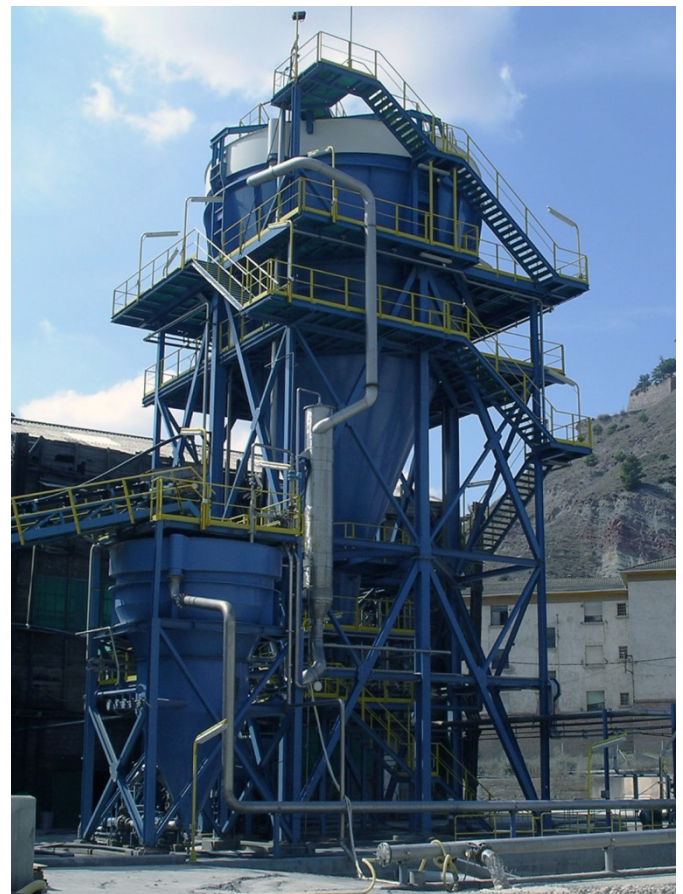
100 t/h HYDROSAL-F2 salt purification plant in Spain
